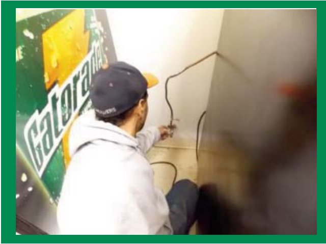
Water lines for the vending machines installed at the Michigan Institute for Public Safety Education
