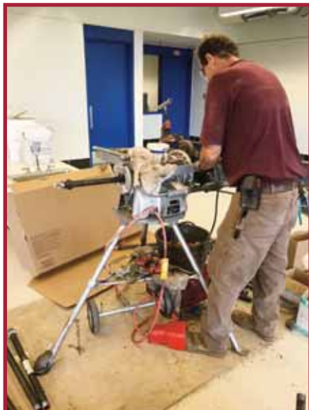
Sprinkler System Updates
