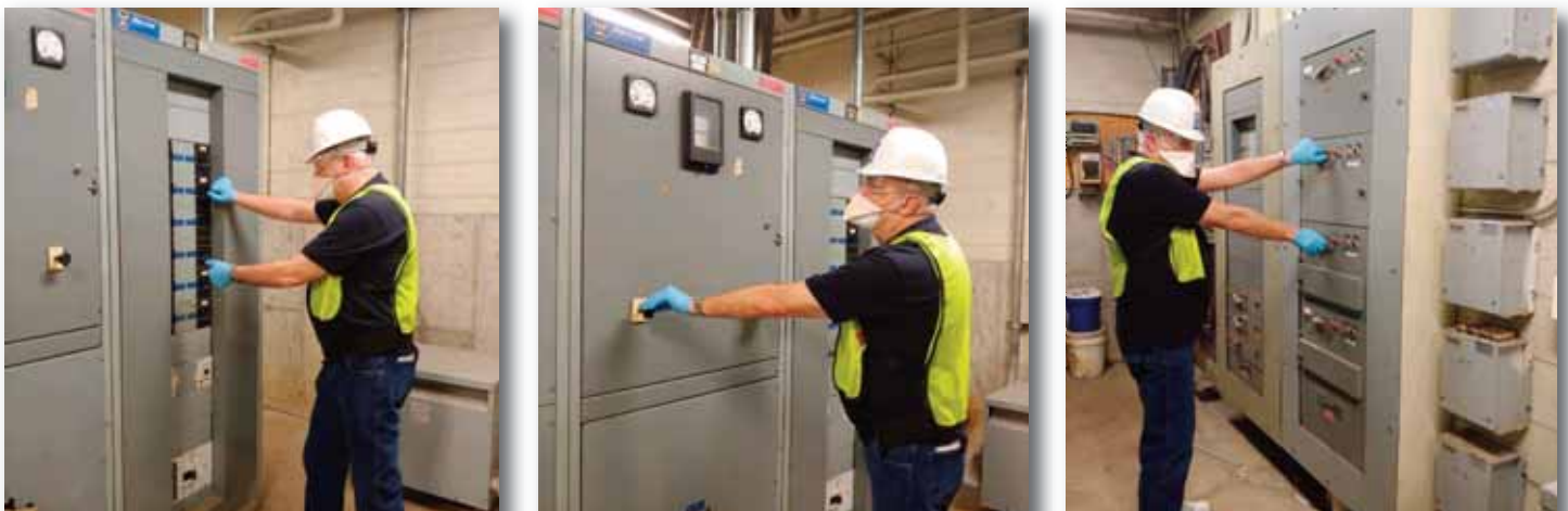
Curtis L. Ivery District Office Building Power Shutdown to Accommodate TCF Center Hospital Conversion
