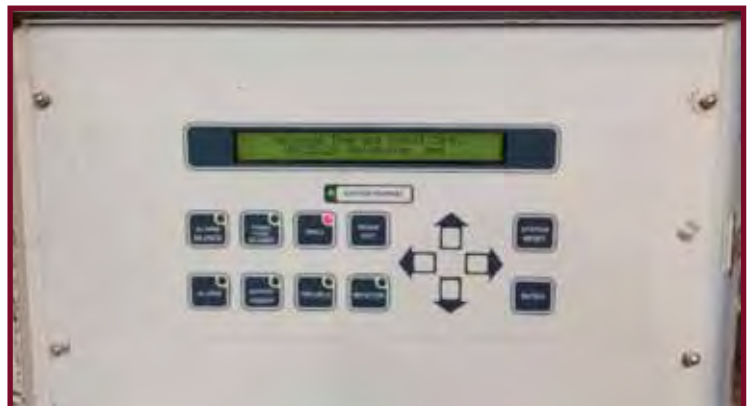
Fire System Test and Inspection at Ted Scott
