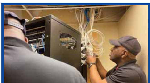
Northwest Campus UPS Battery Installation
