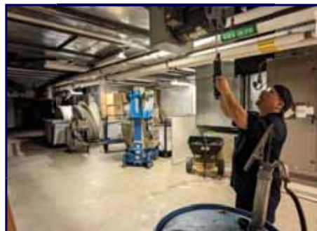
Leo Rocha greases the return motor in the ventilation system at the Ted Scott Campus.
