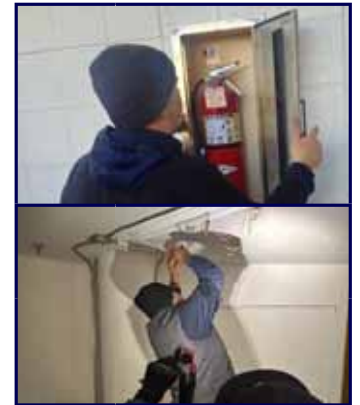
Eastern Campus had a Fire Extinguisher tag inspection and old paint removal from ceiling.
